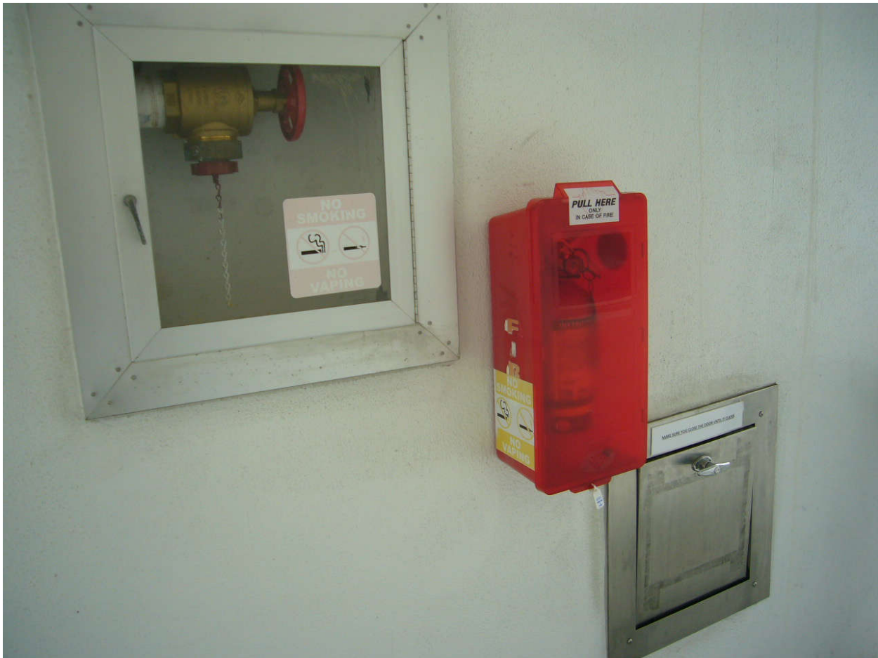
Standpipe, Extinguisher and Trash Drop
