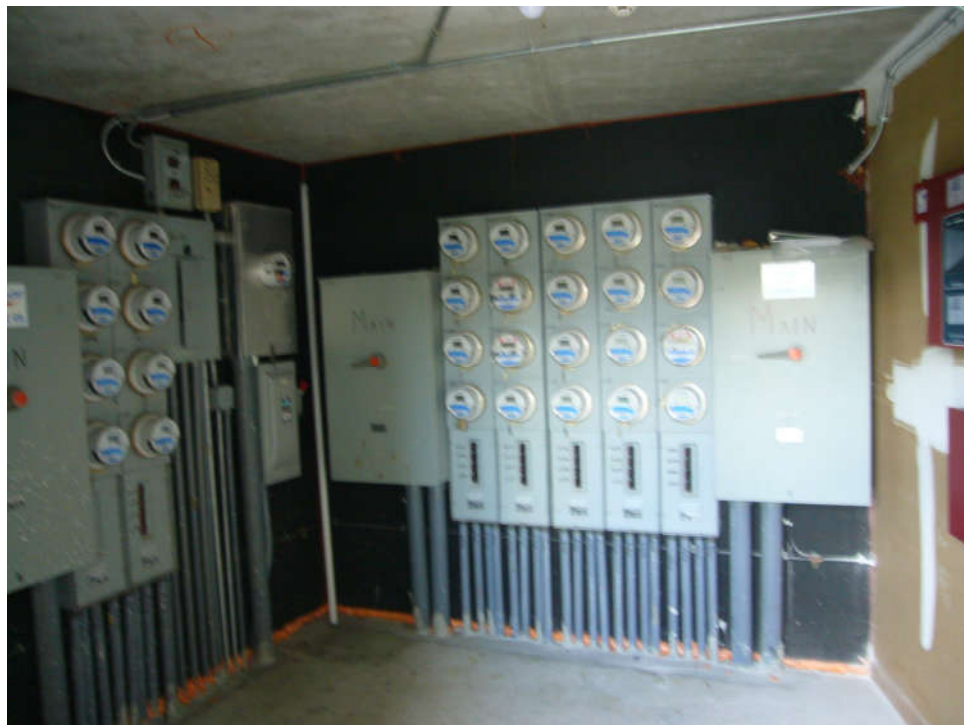
Typical Meter Room
