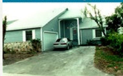
Level 2 - Major damage; habitable
