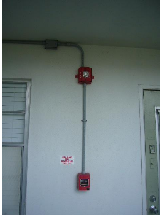
Upgraded Local Fire Alarm System
