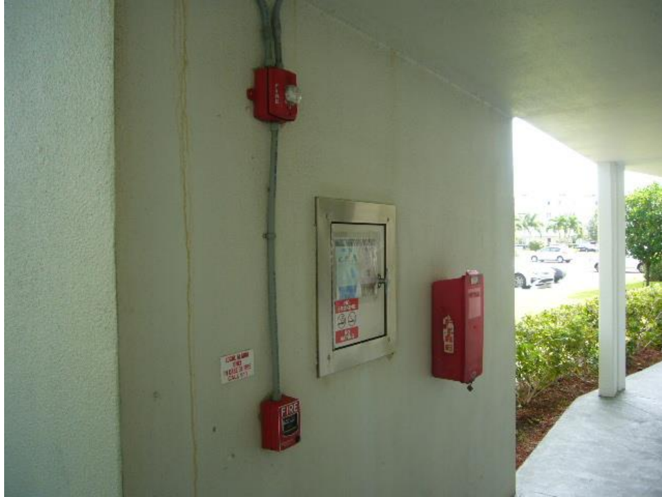
Trash Chute, Local Fire Alarm
