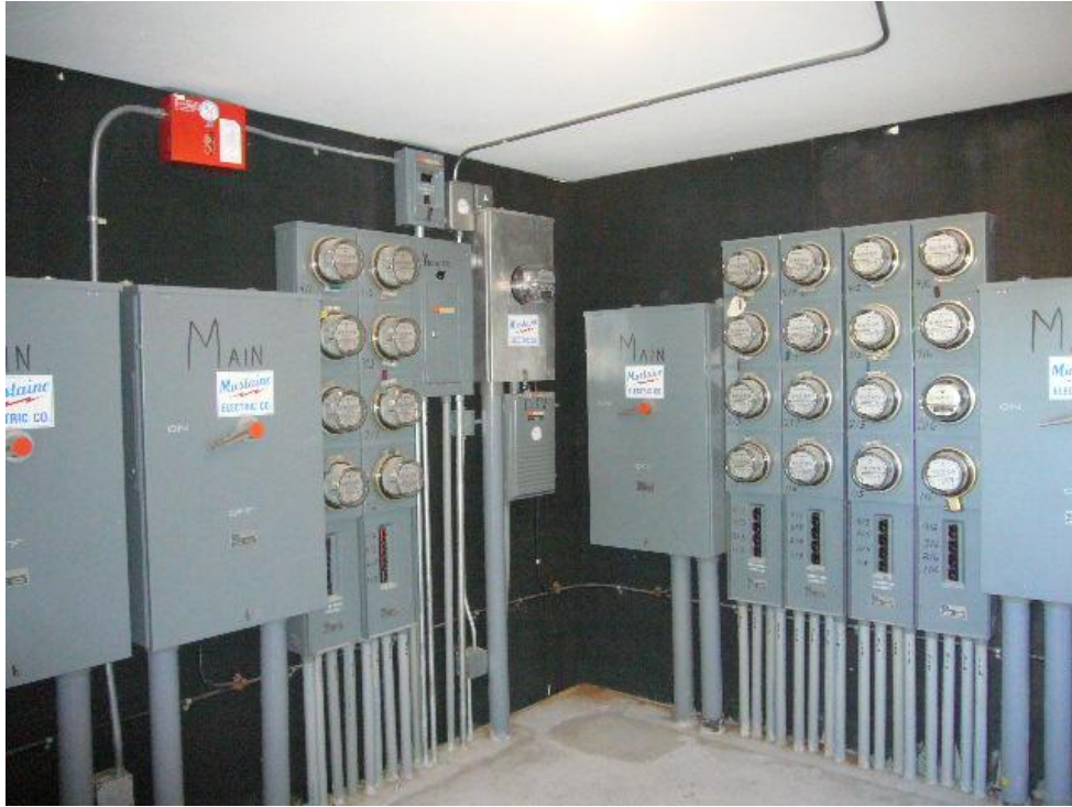
Typical Meter Room
